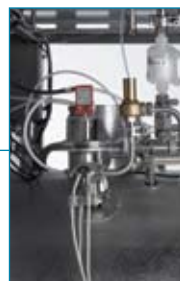
MODULATING VALVE ON FEED STEAM INLET
