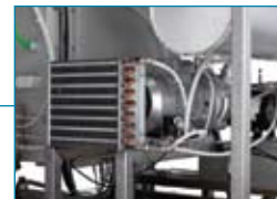
CONDENSATE DRAIN COOLER AND VACUUM PUMP
